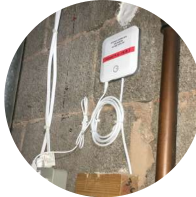
Control HQ Hubs hidden in voids between rooms
