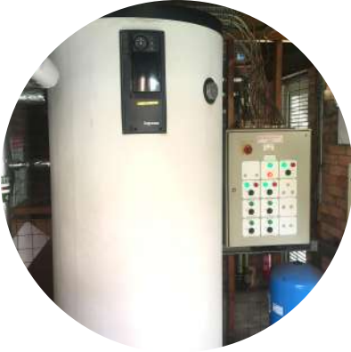
Integrated into BEMS to control local circulation pumps and monitor hot water
